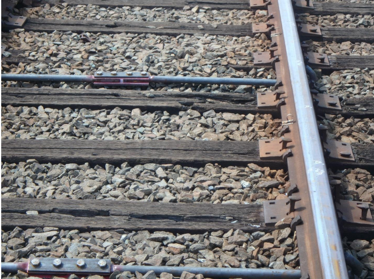
Figure 2. Deteriorated cross-ties at accident location. The gage rods were added postaccident.
