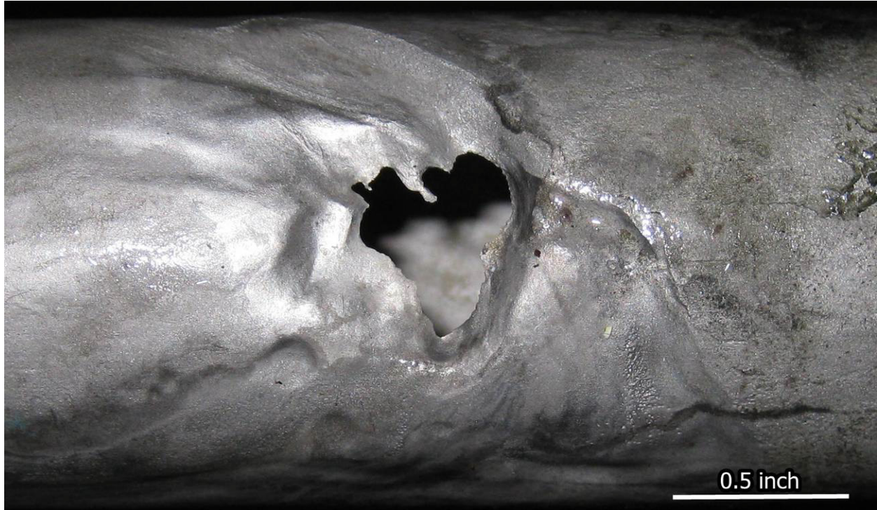
Figure 10. The larger hole eroded from the outside-in on the oleum sample line 26
