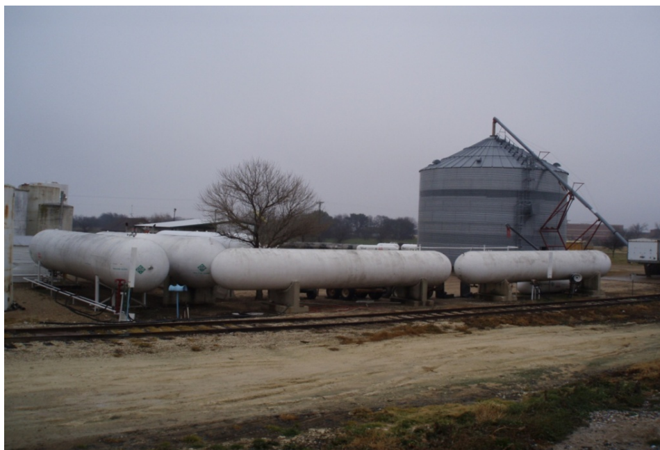
Figure 6. Anhydrous Ammonia Storage (Source: WFC Insurer)
