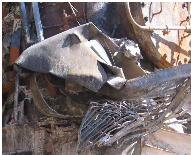
Figure C-4. Residue treater shell fragment lodged in catwalk of adjacent distillation column
