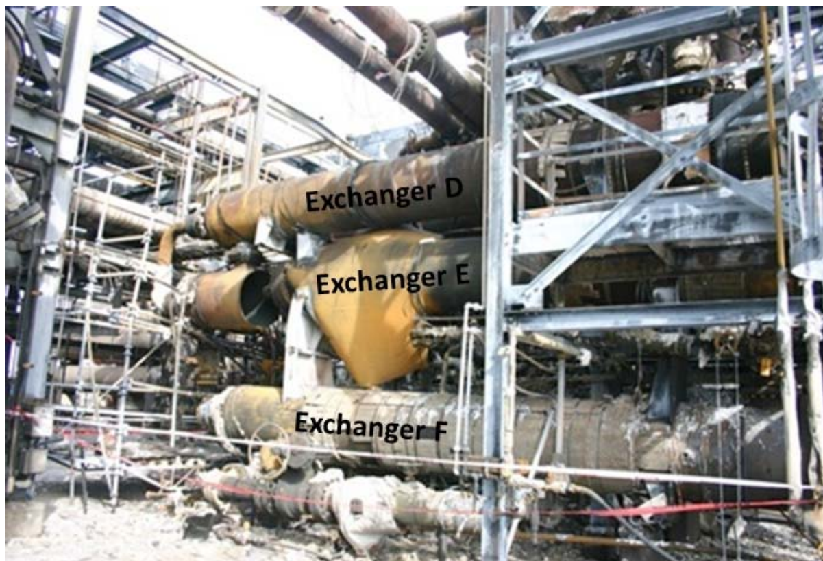
Figure 8. Post-Incident View of D/E/F NHT Heat Exchanger Bank
