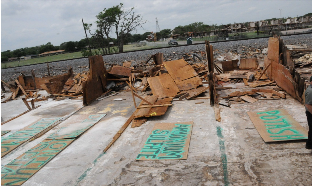
Figure 8. Plywood Bin Wall, Post-Explosion (Source: CSB)
