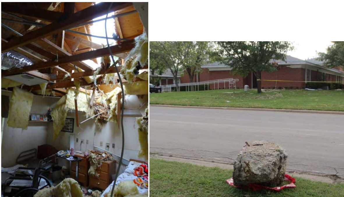
Figure 35. Crater and Debris (left) from Fragment (right) of WFC Facility Foundation that Impacted West Rest Haven (Source: ABS Consulting)
