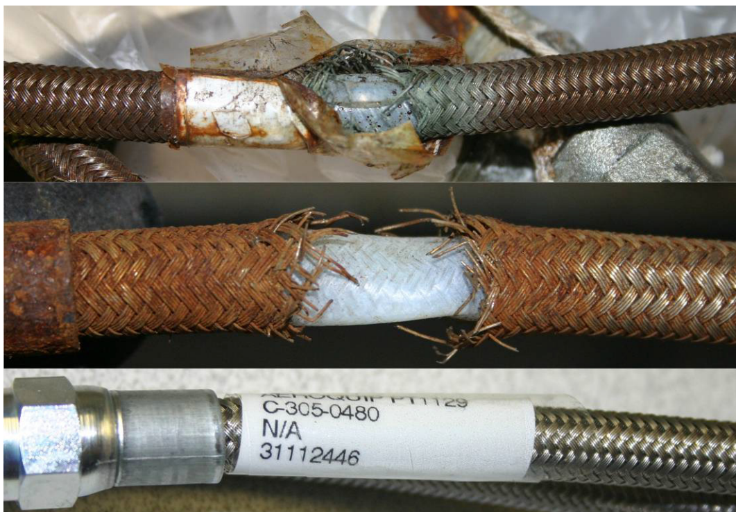
Figure 16. Flex hose comparison photographs: (top to bottom) ruptured riverside hose, flow restricted hillside hose, a new hose with attached ID tag
