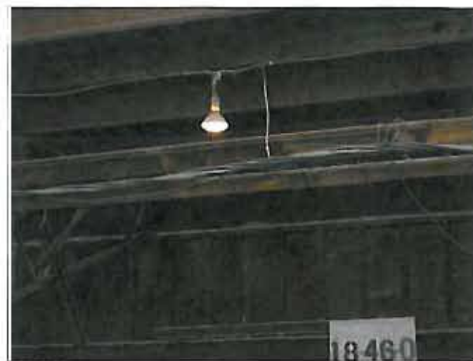
Figure 53. Exposed 440-Volt Electrical Wiring Identified in 2007 Survey (Source: Triangle Insurance Company)
