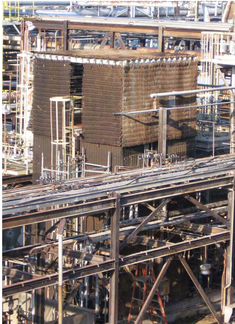
Figure 2. MIC day tank shield blanket structure
