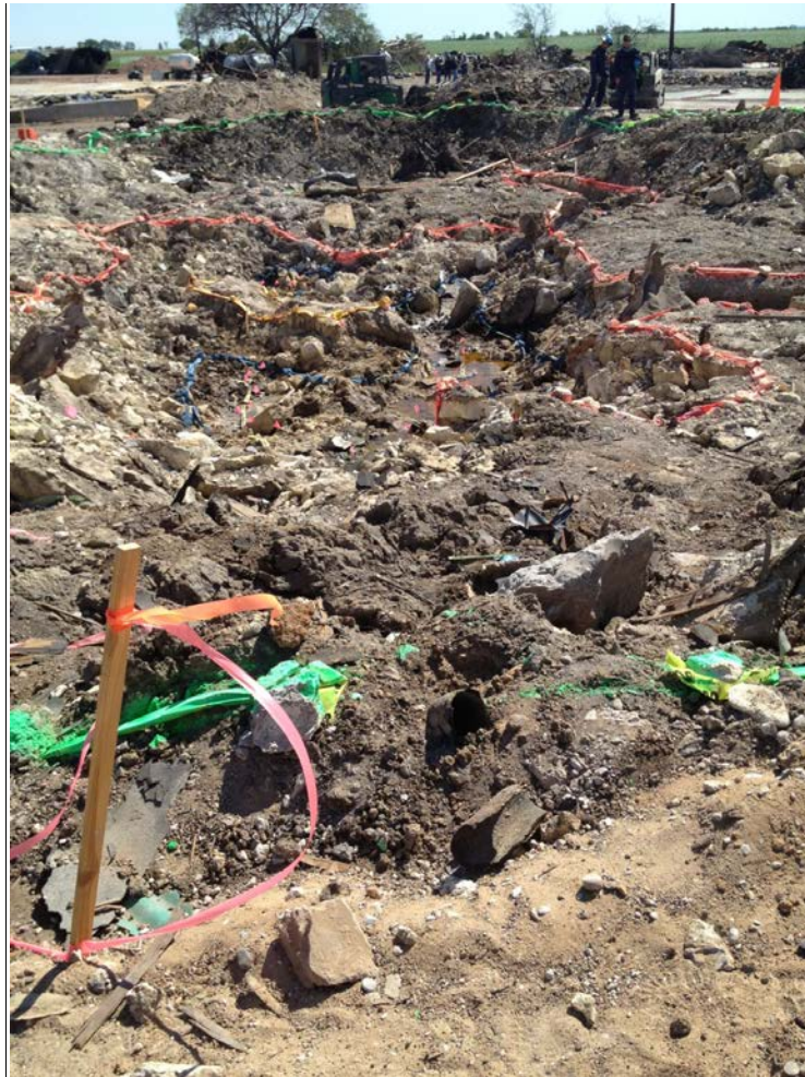
Figure 48. Ground-Level View of WFC Explosion Crater (Source: CSB)
