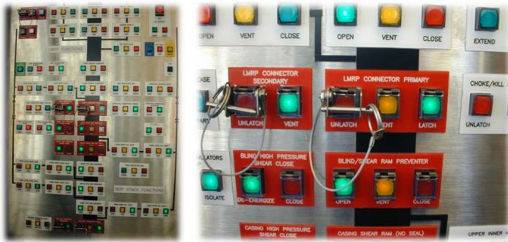
Figure 2-4. Control panel (left) and partial closeup of control panel on the Deepwater Horizon found in the driller's cabin and on the bridge of the rig. These controls are used to activate the BOP. 12
