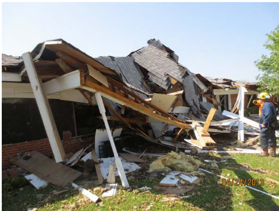
Figure 33. Damage to Reagan Street Entry of West Rest Haven (Source: ABS Consulting)
