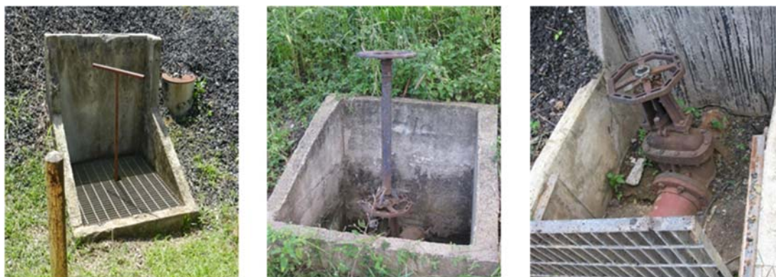
Figure 15: Various dike drain valves at CAPECO. Tank 409 fixed stem dike drain valve (left): position of the valve is undeterminable without physically turning the valve. Rising stem valves (center, right). In some cases, the valve position is hidden in the sump (center).
