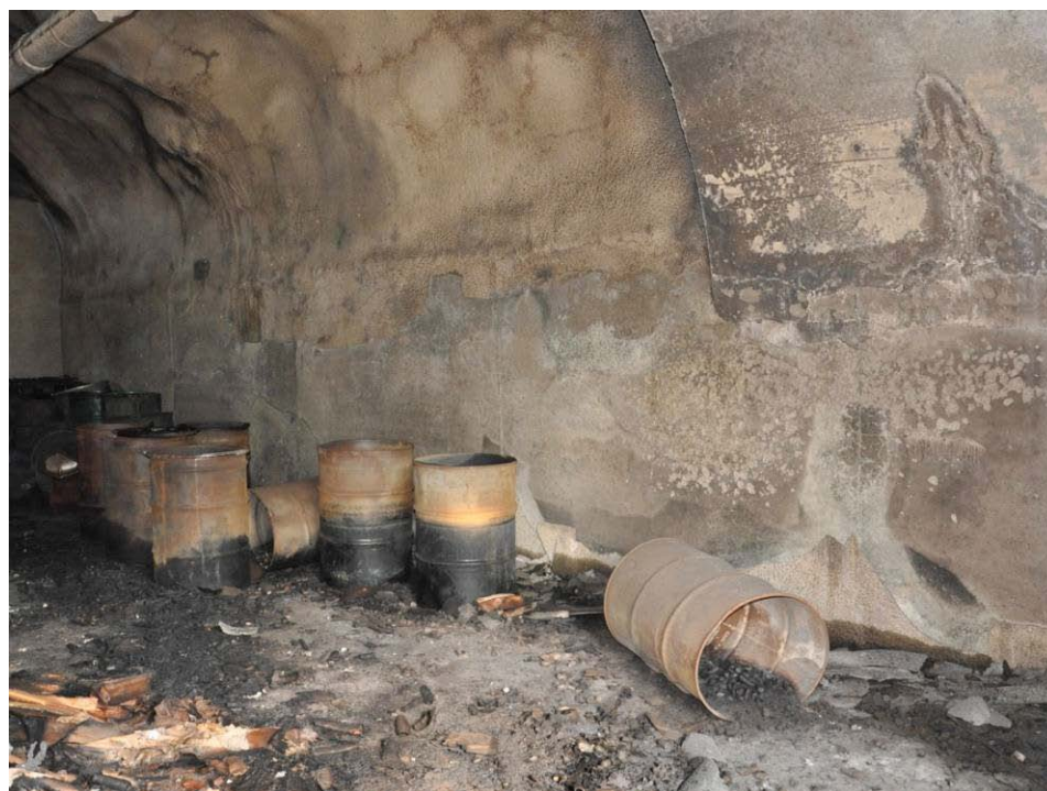
Figure 16. Interior of the magazine post-incident
