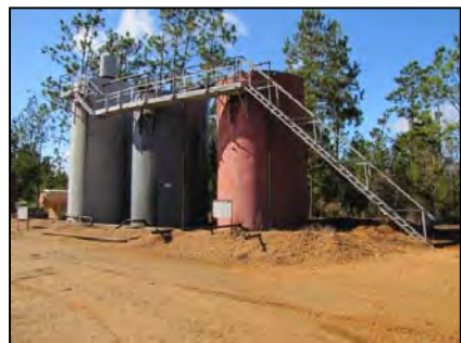
Figure 6-5: Oil and gas production site in Carnes, Mississippi with elevated catwalk
