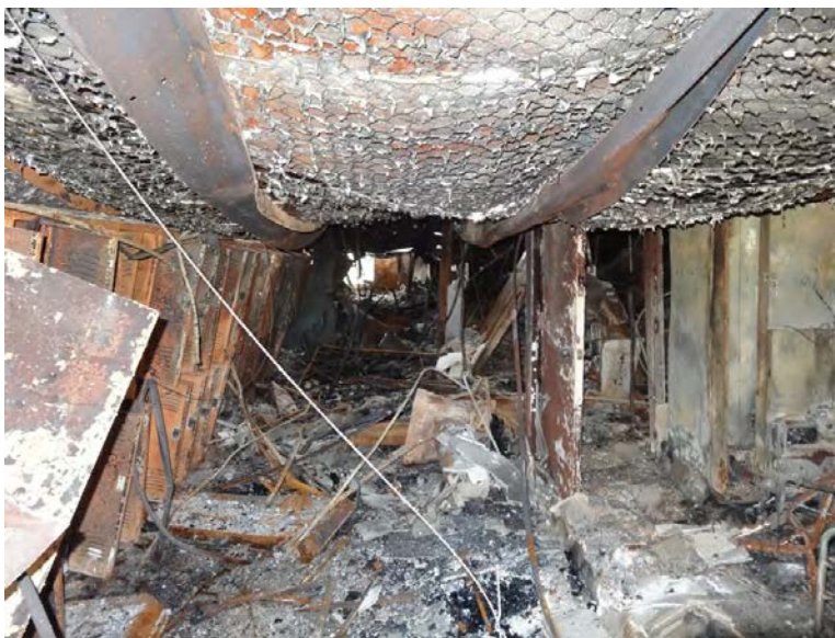
Figure 27. Interior of Burned Northeast Section of WIS (Source: ABS Consulting)
