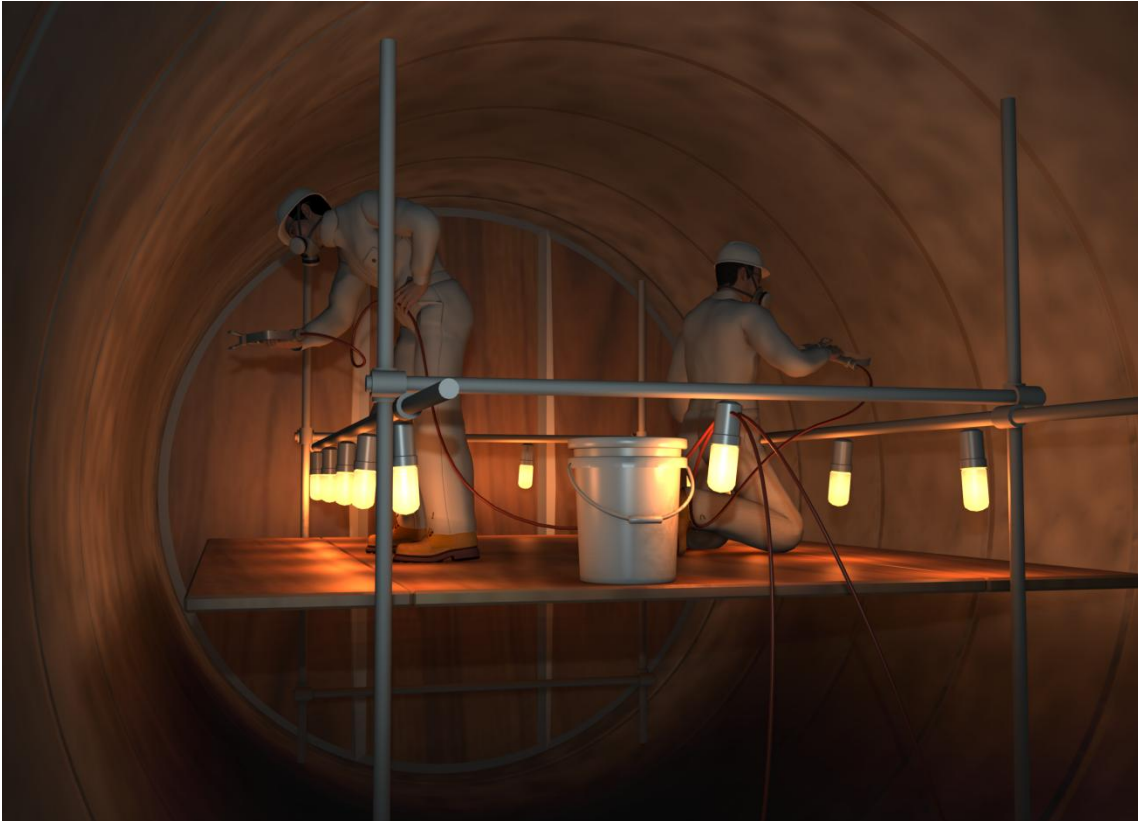
Figure 9. Depiction of contractors recoating the penstock interior near the temporary west bulkhead
