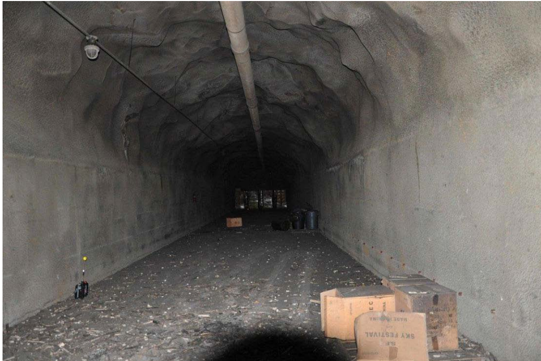
Figure 17. Rear interior of magazine, behind concrete partition, post-incident
