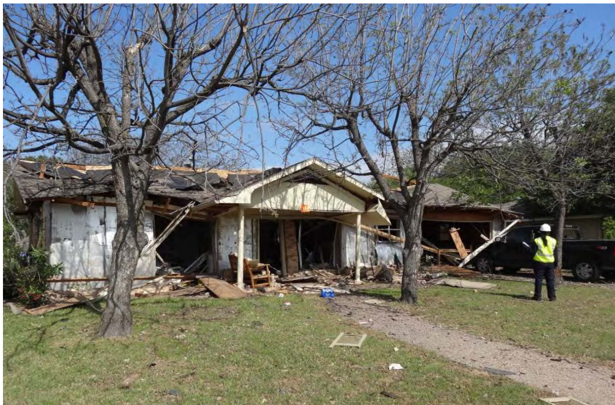
Figure 37. Example of Damage to Single-Family Residential Structure (Source: ABS Consulting)
