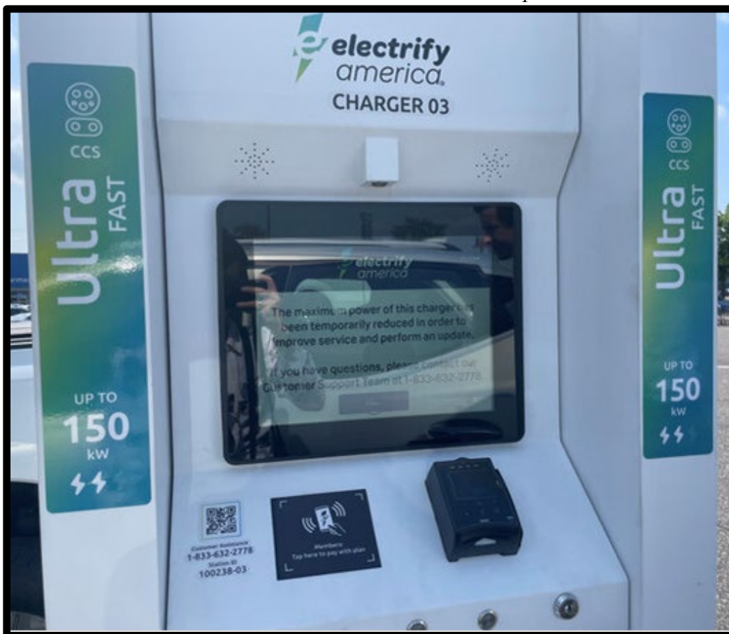
Figure 7: An EV charging station reads “The maximum power of this charger has been temporarily reduced in order to improve service and perform an update” on DOE Secretary Granholm’s summer 2023 EV road trip 127
